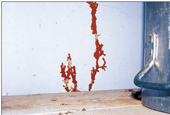
Figure 7. — Termite shelter tubes.
